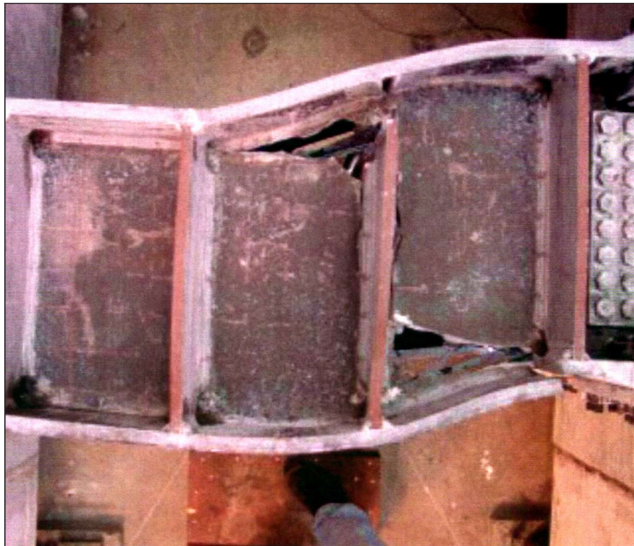
Web Fracture of Shear Link at 0.15 rad
