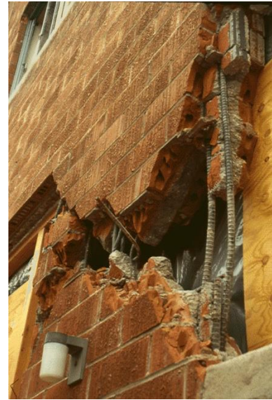
Figure 4-2. Damage of R/M Building in
