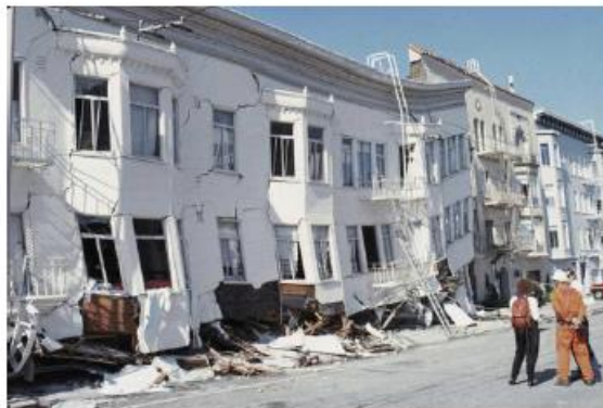
Figure 1. Soft-story building collapse in the 1989 Loma Prieta Earthquake.
