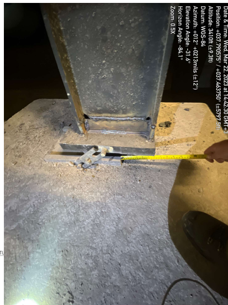
Residual offsets at pipeline supports
